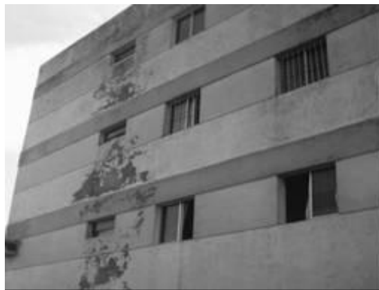
Figure 2. Building 05 facade with painting wear.
