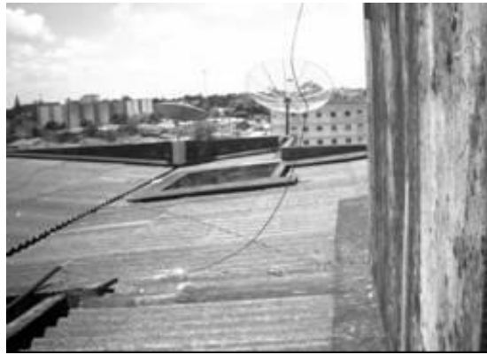
Figure 1. The view from Building 04 deck - Lack of impermeable cover in several parts of the deck.
