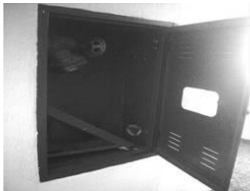
Figure 8. Fire hose cabinet without fire-fighting hose in Building 04.
