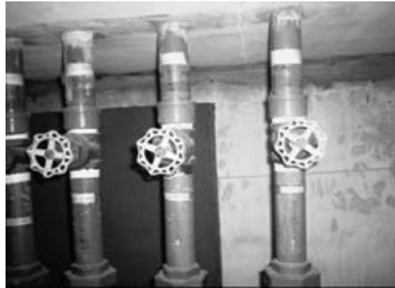
Figure 3. Barillet with identified columns in Building 09, facilitating maintenance operation.
