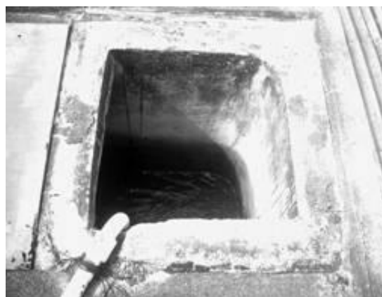
Figure 5. The opening edge of the top reservoir in Building 09 with pieces of iron.
