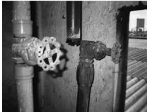
Figure 7. Fire-fighting water supply column broken in Building 02.
